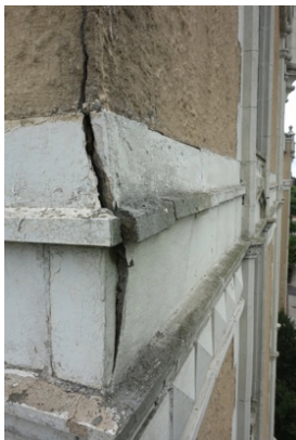
Terra cotta cracked and buckled outwards because rebar behind it severely rusted. The mortar had deteriorated to sand.
