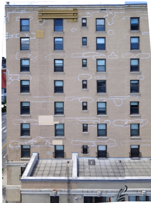
There was no time for a survey and report. We circled the loose pieces of stucco with spray paint, and repairs followed immediately after.
