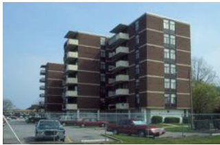
The original construction had concrete floor slabs exposed at the edges, a source of chronic leakage
