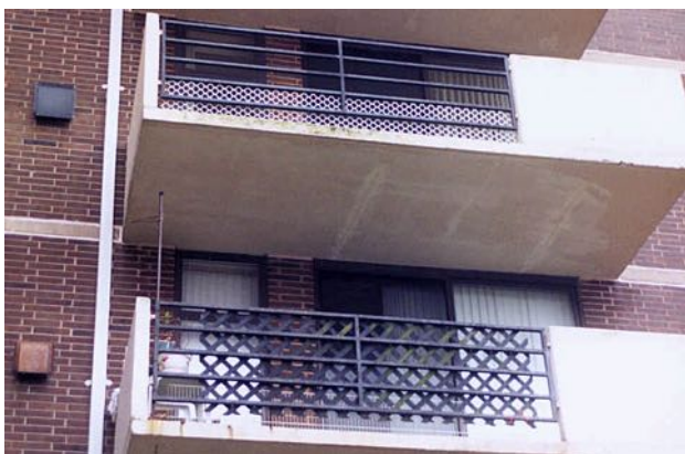
Management had been "child-proofing" individual balcony guardrails as best it could. These rusted guardrails were replaced with new galvanized steel as part of the re-cladding.
